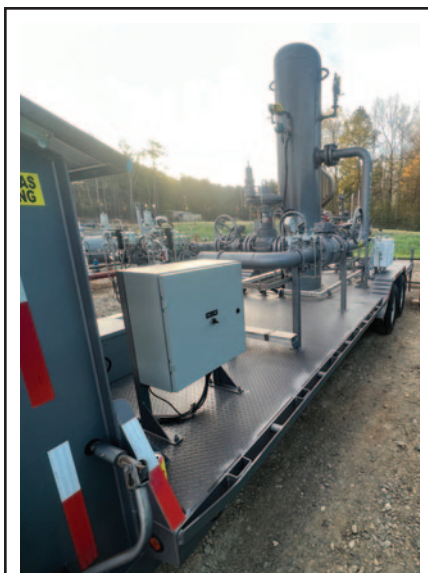
This gas conditioning skid from ProFrac Services is enabling a hydraulic fracturing fleet to run on field gas by removing contaminants such as liquids, condensates and chemicals. These skids may become more common as the industry looks for ways to use stranded gas.
